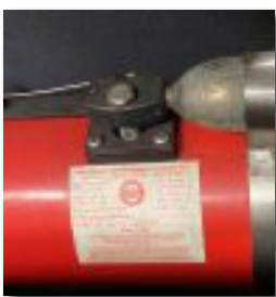
With no date and a hard to read serial number, this will need to be replaced.
